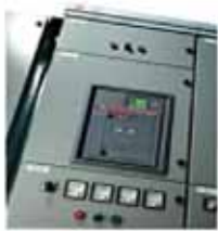
Faults: no problem
